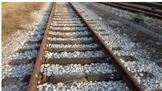
Figure 2. A cracked sleeper
