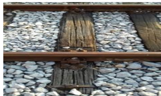
Figure 3. A cracked sleeper
