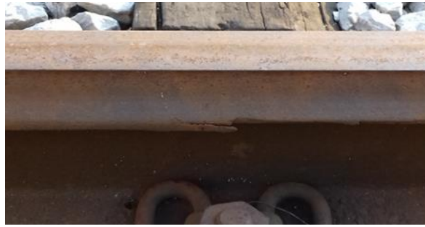
Figure 1. A worn-out rail.
