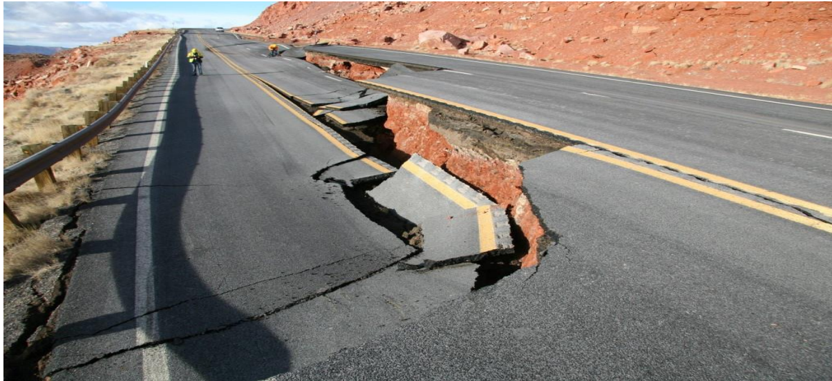
Fig.1 Damage to the road due to landslides
